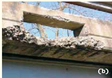
Figure 4. Old Bridge 14802301, Greene County, MO: degradation of concrete deck and steel girders (a), and of safety appurtenance (b).
