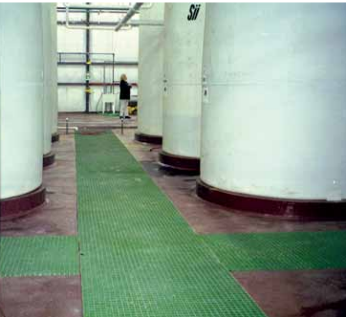
The Exide Battery Plant in Manchester, Iowa installed corrosion resistant DURAGRATE® around its tanks of sulfuric acid.
