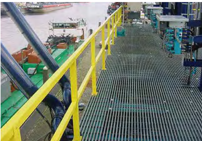
Liquids ship loading facility incorporates low maintenance DURADEK® grating and SAFRAIL™ handrail system.
