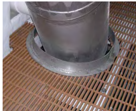
An 850mm stainless steel pipe sleeve is used on a NORSOK required pipe penetration.
