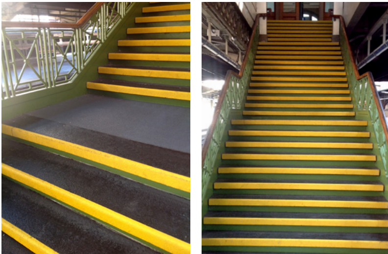
These rail station stairs in Baltimore, MD were renovated with DURATREAD™ stair tread covers, allowing the train station to keep the existing stairs, reduce downtime, and saver time and money in the process of the upgrade.
