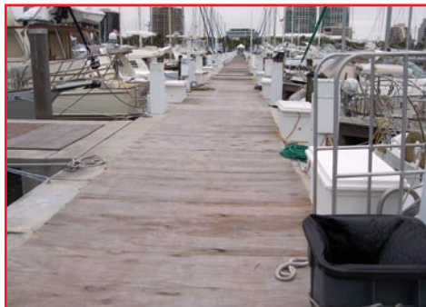
Rotting wooden planks were a problem at Dinner Key Marina before Strongwell's DURAGRID® pultruded grating was installed.
