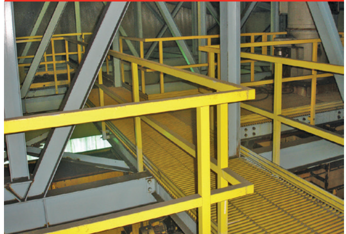
Fiberglass: 16+ Years Exposure
