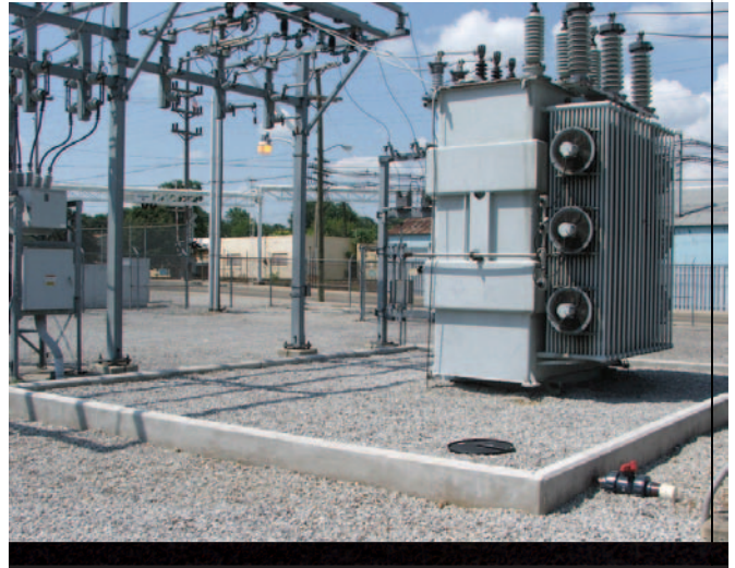
A traditional concrete oil-containment system used around one of AEP's substations.
