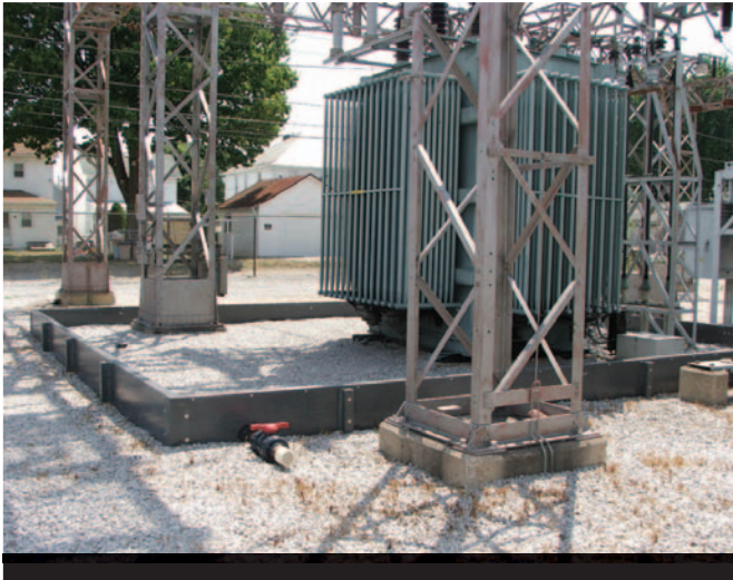
Composite-panel system installed for oil containment around an AEP substation transformer.
